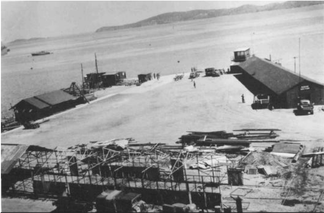
Expansion of the Marine Section capability in 1942 is clearly evident by the construction of facilities in the fore ground. ( J. Hewett)
